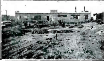
Grading foundation for the new power house, galvanizing and iron stock at the plant on E. Eldorado
