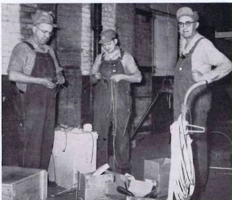
As this issue goes to press, work on the new office expansion at our main plant is well underway. Above, three electricians begin the rewiring. They are, left to right, Carl Smith, Robert Ridgeway and John M. Smith, foreman. The expansion will add the much needed space to our now crowded office facilities. Moving to the new section will be all of Accounting, Department Billing, General Accounting, Accounts Receivable, Credit, and Troy Roush and Bud Levey of the Sales Division. Augie Werdes, plant controller, will move to a new office in the new section. On the other side, a partition will be erected separating the Sales Division and Headquarters. New offices will also be built for Don Radcliffe and Harlan White.
