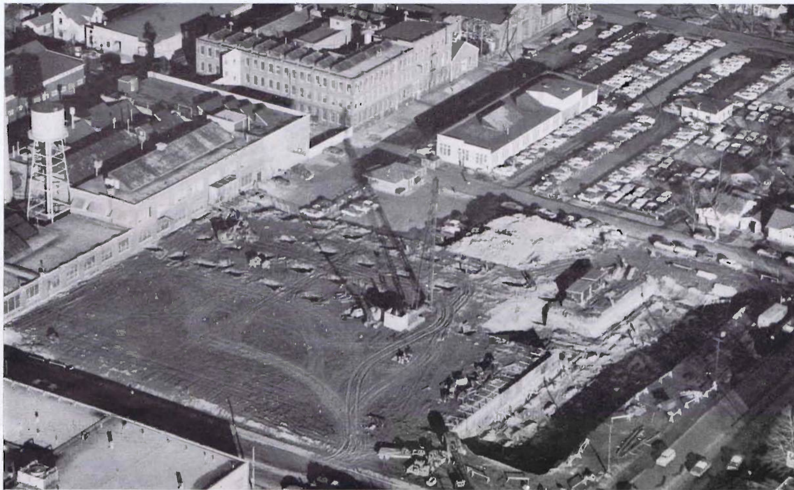
The afternoon sun casts long shadows on the construction site in Decatur. In the lower right corner, the walls are being poured for the new office building. In the center, the holes show the places where piling are being driven. The shadow of the pile-driving rig falls
