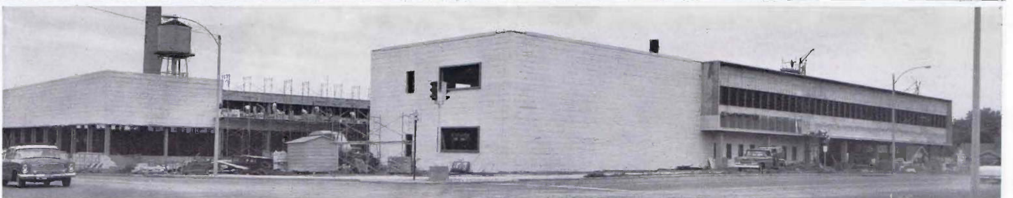
The Mueller Co. expansion in Decatur is about 50 per cent finished and plans are being made for a move into the new office in December. Since this picture was taken the sun shades have been put on the front windows, most of the brickwork completed
