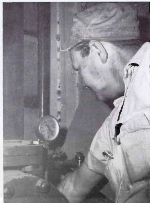
"How much" pressure in the plant's sprinkler system is shown by this clock as W. J. Hixon, Maintenance Foreman, makes a regular check.
