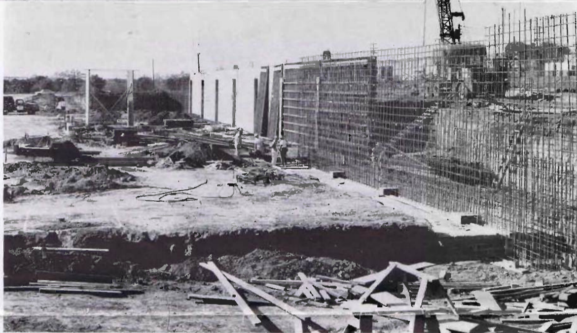
Rising in the midst of the hills of Southern California is the new Mueller Co. plant at Brea. The upper photo shows a retaining wall under construction as seen from the rear of the factory area. The area where the equipment is working, now has a
