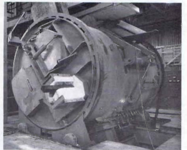
One of the electric melting furnaces with a 60-ton capacity.
